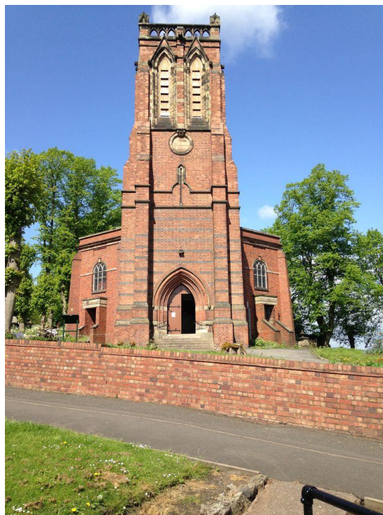
The tower today with pepper pot removed. Note space for clock dial below bell openings.
